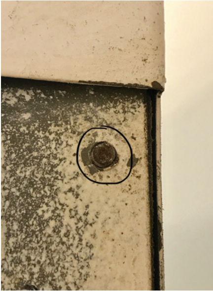
Figure 6. The top screw on the door leaf was broken off.
