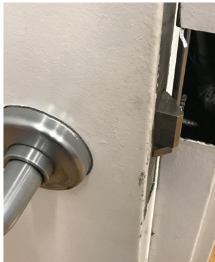
Figure 13. The closer should be adjusted so that it will close and latch the door positively even when it's barely open.
