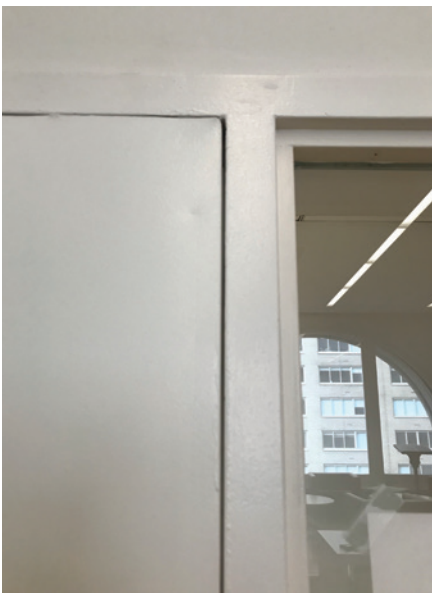
Figure 9. Shown is the point where the door was rubbing.
