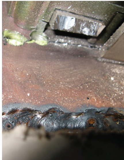
Figure 9. How did the bolt get cut off by just the two holes to the left of the bolt?
