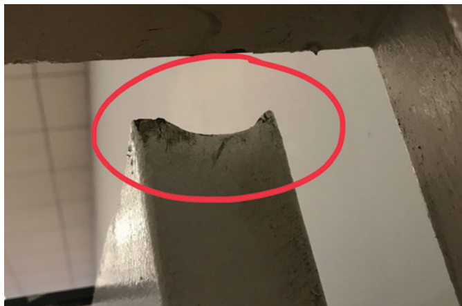
Figure 4. The indentation within the red circle was caused by a broomstick or wedge propping the door open.
