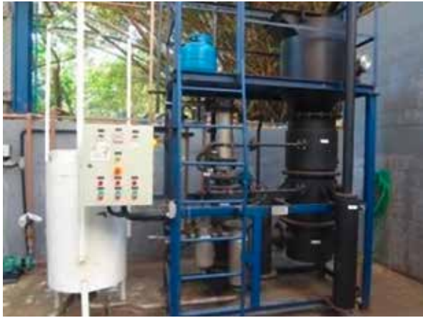
Gasification pilot plant at UFBA [3]
